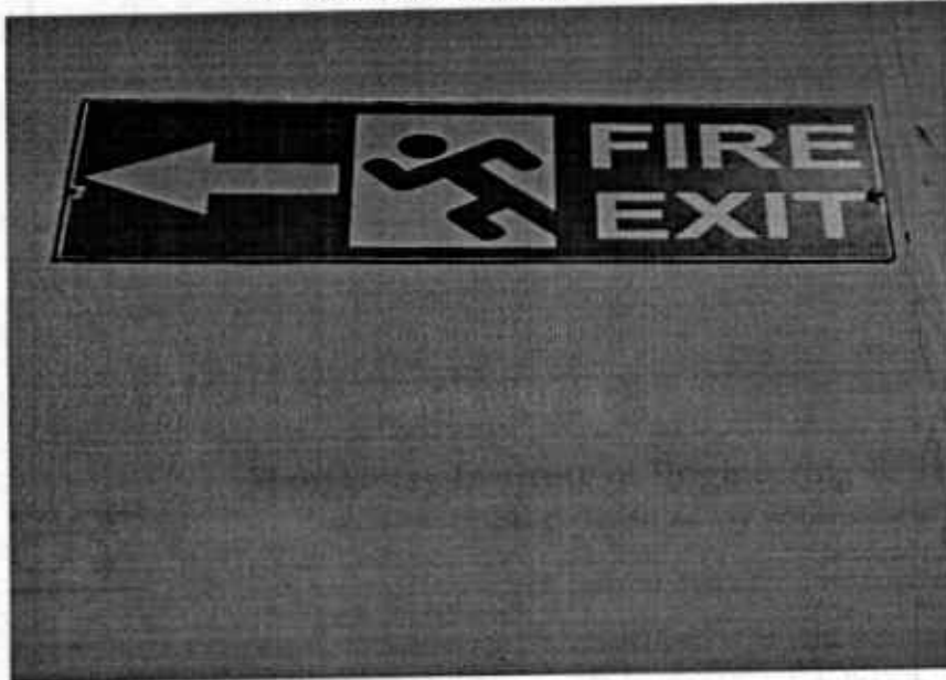
Fire Exit Third Floor Right side
